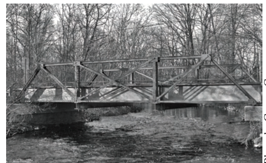
Vernoy Rd Bridge over S. Branch Raritan River, Lebanon, Tewksbury and Washington Twp
